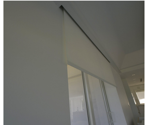
Shade edge tracked to the raked gable ceiling.
